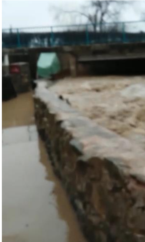
Image 2. Extract from local residents' video showing water levels across the wall at the downstream end at the approximate peak river level.
