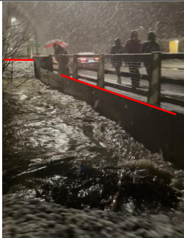
View of the fire station road crossing and bunded area. Note the difference in level (shown in red) between the top of bund and bridge threshold
