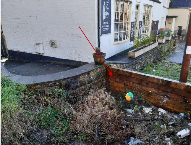
Figure 10: Wrack mark at stop logs (Source: NRW staff)
